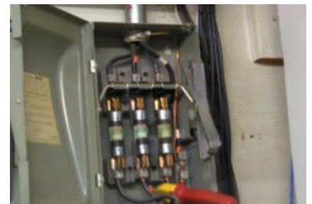
This image shows a typical disconnect box. When observed by the naked eye, nothing appears to be wrong.
