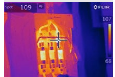
This is the thermal image of the same disconnect box. Note the abnormal heat level on the fuse clip.
